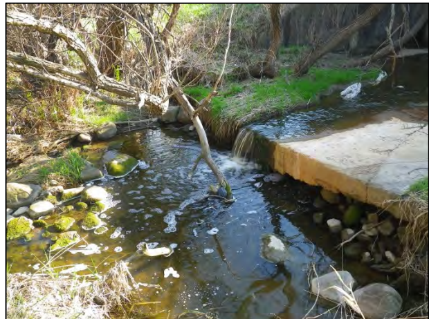
Looking north along the tributary outlet of Innisfil Creek from east (downstream) of Highway 400 (Wilson Drain). Note barrier to fish
