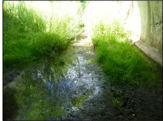
Looking upstream (west) along a tributary of Innisfil Creek from west of Highway 400 (Wilson Drain).
