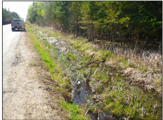
Crossing H: Looking west from north (upstream) of 6 th Line at a Tributary of Banks Creek.
