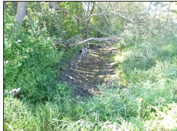
Crossing C: Looking south (upstream) from the southeast quadrant of 6 th Line and Sideroad 5 of the southerly Tributary of Innisfil Creek.
