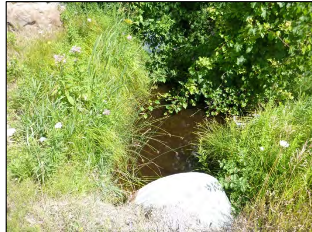
Crossing F: Looking north (upstream) from 6 th Line at a Tributary of Innisfil Creek.
