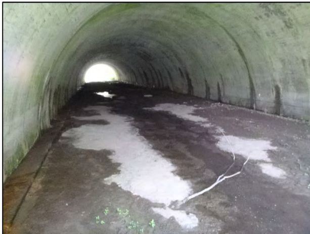
Looking downstream (east) along the tributary crossing of Innisfil Creek from west of Highway 400 (Wilson Drain).
