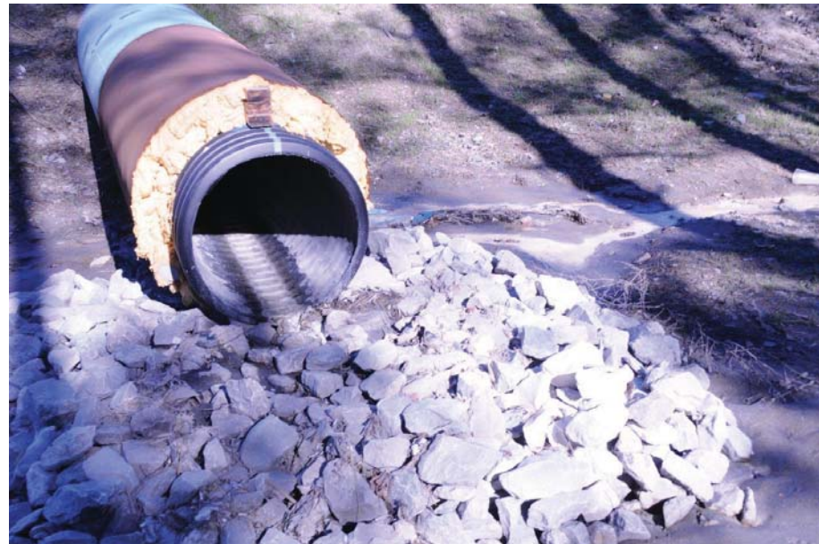
Photo 4: Area of stained soil located west of Highway 400, view eastward
