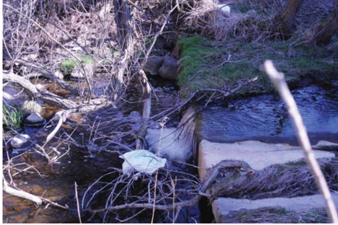
At the downstream end of the concrete arch culvert the stream drops 300 cm from the base slab
