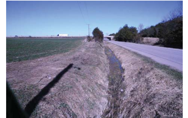
North ditch of 6 th Line west of Highway 400 (in distance) conveying runoff from MTO culvert C-56 just north of the intersection
