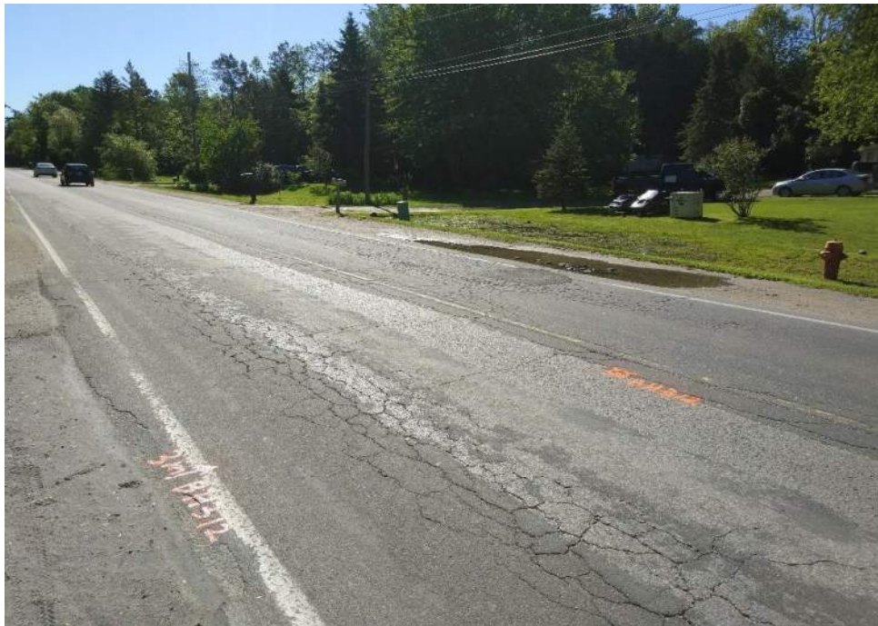
Photograph 12 – 7 th Line, looking east, 110 m west from Wingrove Avenue, showing moderate to severe alligator cracking, slight to moderate longitudinal and transverse cracking, moderate edge cracking, slight patching, and slight depression. It was noted that water ponded on the south side shoulder area.
