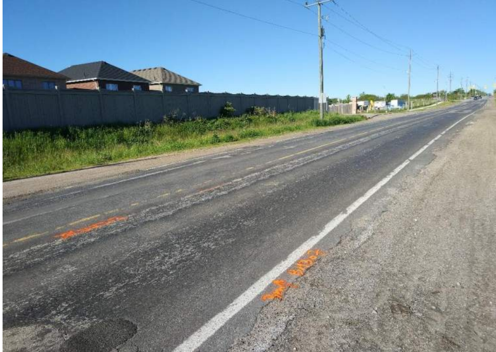
Photograph 7 – 7 th Line, looking west, 210 m east from Webster Boulevard, showing moderate pavement edge broken and slight patching.
