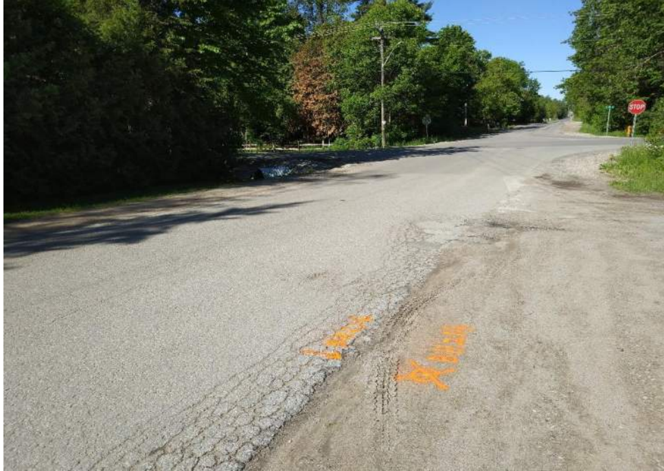
Photograph 15 – 7 th Line, looking west, 36 m east from St Johns Rd, showing severe alligator cracking, severe pavement edge broken, slight longitudinal cracking, moderate patching and moderate weathering.
