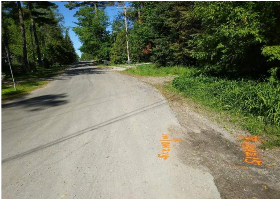
Photograph 16 – 7 th Line, looking west, at intersection of Cross Street, showing slight edge cracking.
