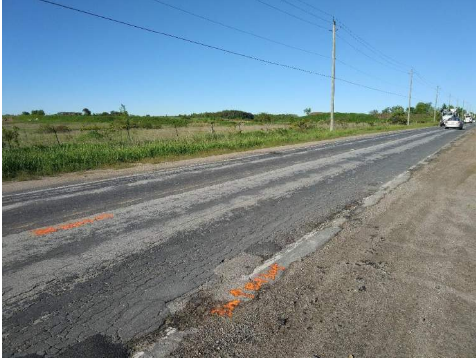
Photograph 5 – 7 th Line, looking west, 175 m west from Webster Boulevard, showing severe alligator cracking, severe pavement edge broken and slight patching.
