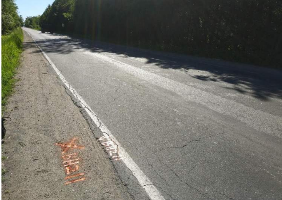
Photograph 11 – 7 th Line, looking east, 25 m east from Quarry Drive, showing slight to moderate longitudinal and transverse cracking and moderate to severe edge cracking.
