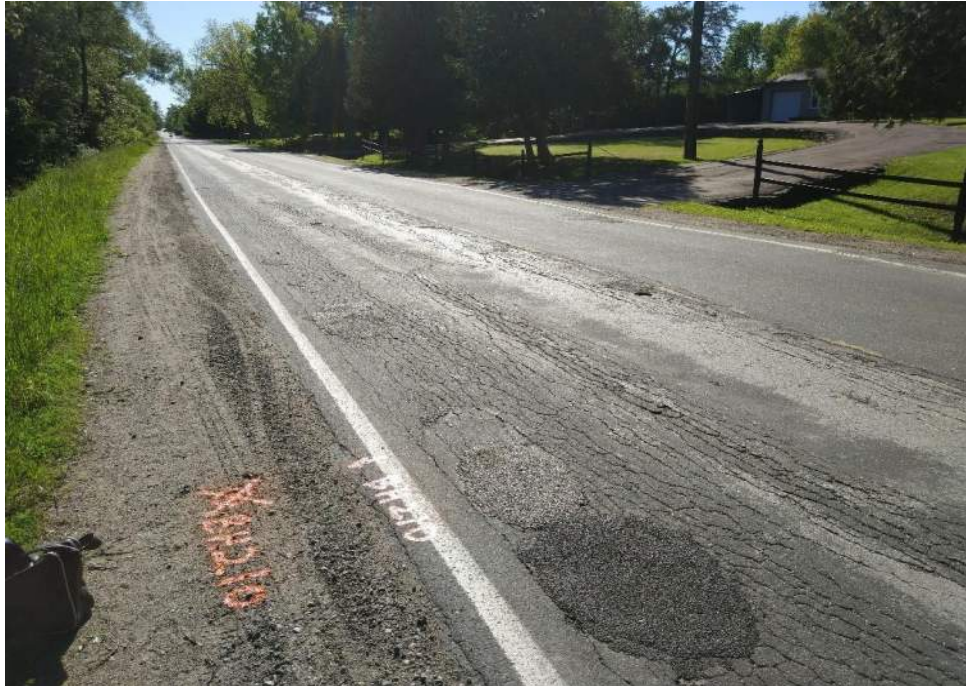
Photograph 9 – 7 th Line, looking east, 170 m west from Quarry Drive, showing severe alligator cracking, slight edge cracking, slight patching, and slight pothole.
