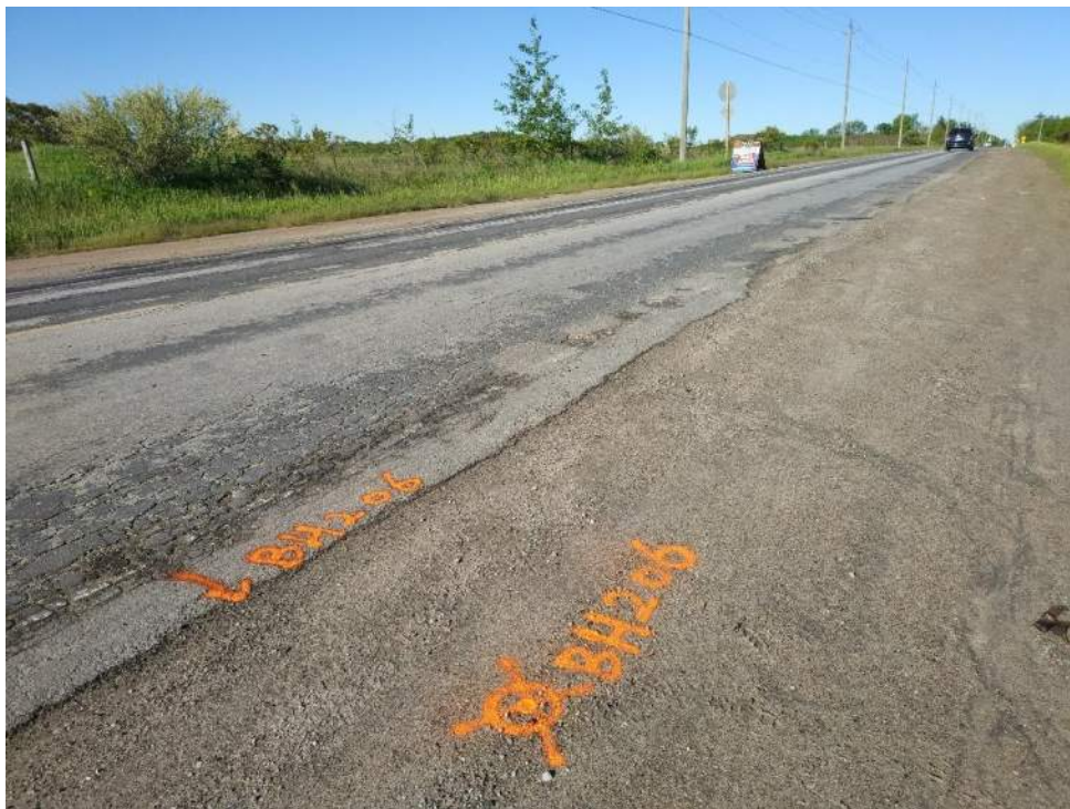
Photograph 6 – 7 th Line, looking west, 80 m west from Webster Boulevard, showing severe alligator cracking, severe pavement edge broken and cracking, and slight patching.
