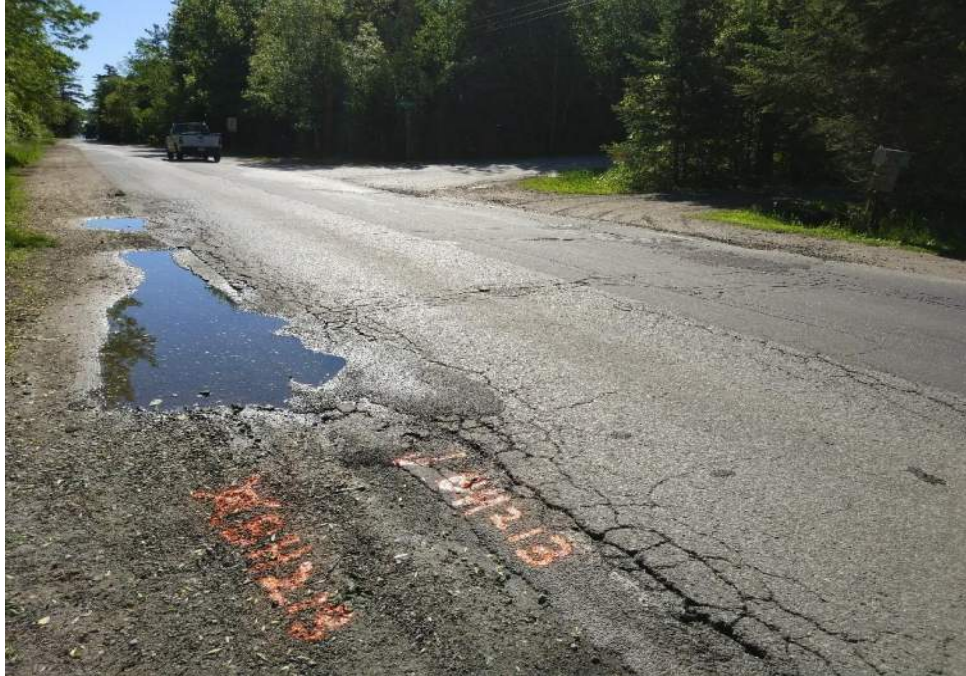
Photograph 13 – 7 th Line, looking east, 10 m west of Wingrove Avenue, showing severe alligator cracking, severe longitudinal and transverse cracking, severe edge cracking, and slight to moderate patching. It was noted that water ponded on the south side shoulder area.
