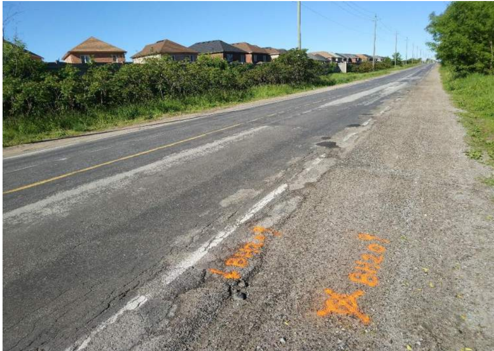
Photograph 8 – 7 th Line, looking west, 385 m west from Quarry Drive, showing severe edge cracking and severe pavement edge broken, and slight patching.
