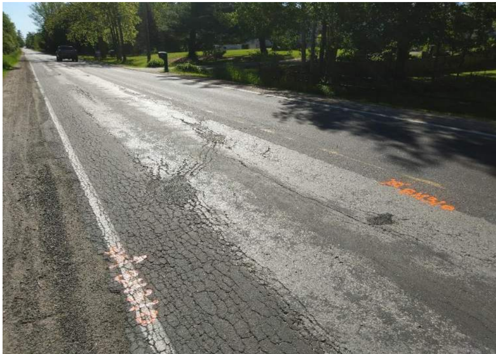
Photograph 10 – 7 th Line, looking east, 80 m west from Quarry Drive, showing severe alligator cracking, severe pavement edge broken, slight longitudinal cracking and slight patching.
