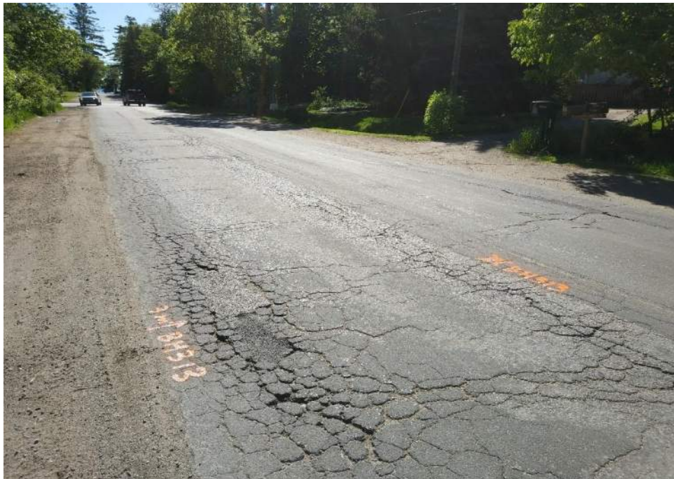
Photograph 14 – 7 th Line, looking west, 75 m from St Johns Road, showing severe alligator cracking, severe longitudinal and transverse cracking, slight edge cracking and slight patching.
