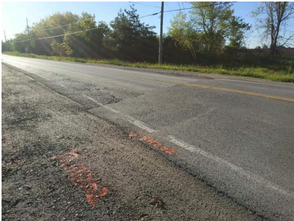
Photograph 2 – 7 th line, looking east, 240 m east from 20 th Sideroad, showing moderate to severe alligator cracking, moderate construction joint cracking, slight transverse cracking, and slight pothole.
