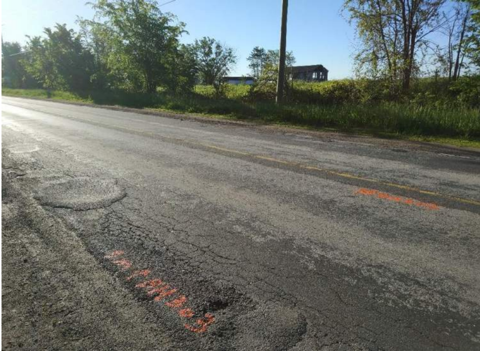
Photograph 3 – 7 th line, looking east, 325 m west from Fox Hill Street, showing severe alligator cracking, slight patching and slight pothole.
