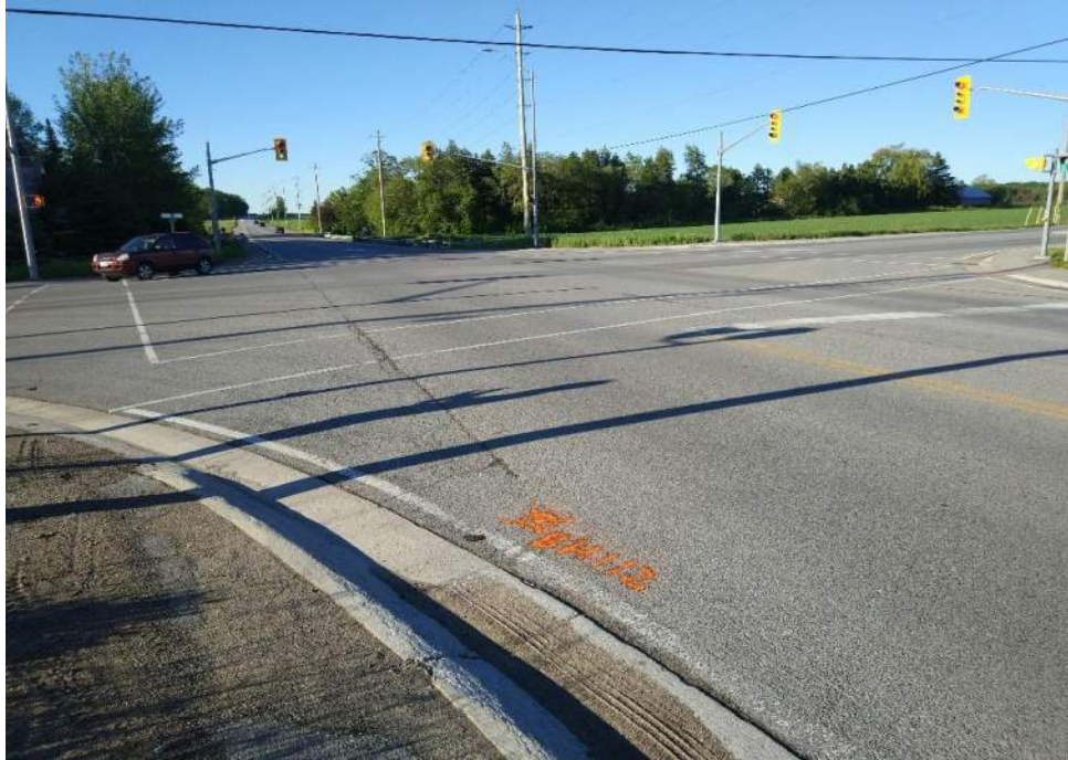
Photograph 1 – 7 th Line, looking south, at intersection of 20 th Sideroad, showing moderate construction joint.
