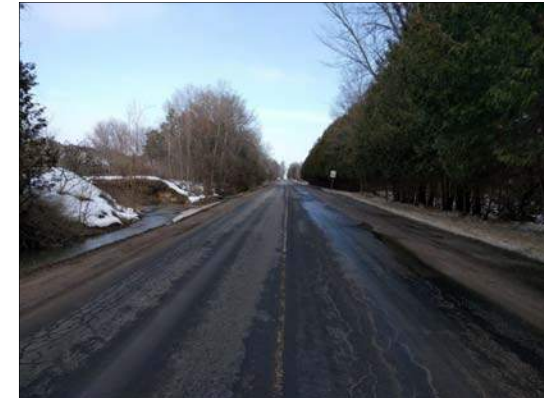
Existing Pavement Structure Deterioration
