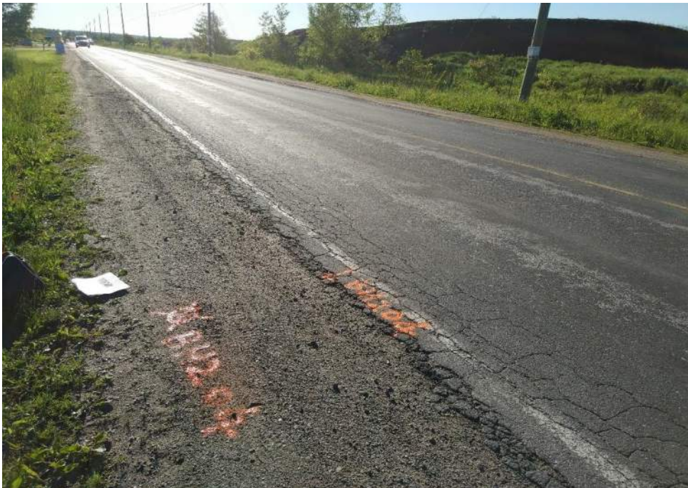
Photograph 4 – 7 th line, looking east, 140 m west from Fox Hill St, showing moderate to severe alligator cracking and severe pavement edge broken.
