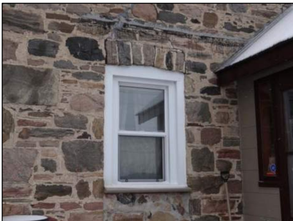
Plate 5: North window on the west elevation. Note the stone infill under the window when it was converted from a door.
