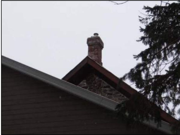
Plate 9: Internal brick chimney at peak of gable end on east elevation, looking west.
