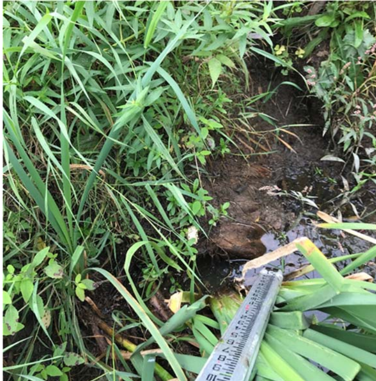
Photograph 16: Obstructed inlet of 600 mm Dia. Buchanan Street/Crystal Beach Road Culvert
