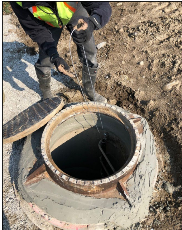
Photograph 16: Technician Removing Pressure Transducer for Monthly Data Download
