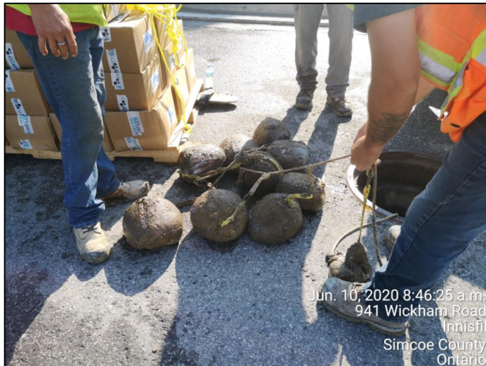
Photograph 14: Removal and replacement of spent Gel Flocculant Blocks
