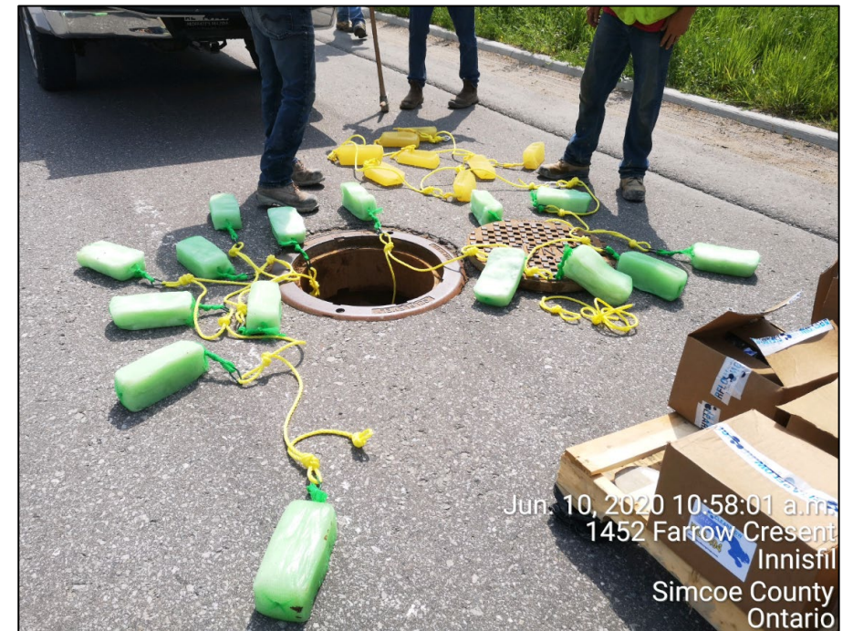
Photograph 3: Installation of Gel Flocculant Blocks (WLB 494 and WLB 360) in a MH structure upstream of SWMF 6
