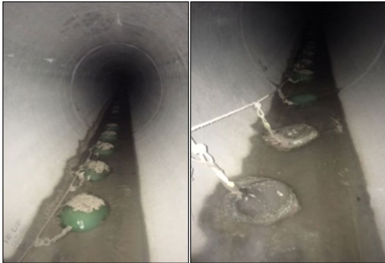
Photograph 12: Fully spent Gel Flocculant Blocks
