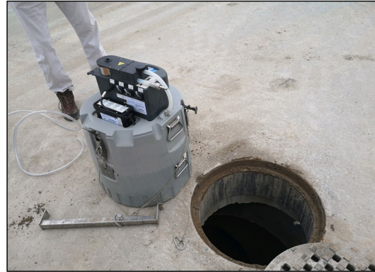
Photograph 23: Preparing Autosampler Device for Installation
