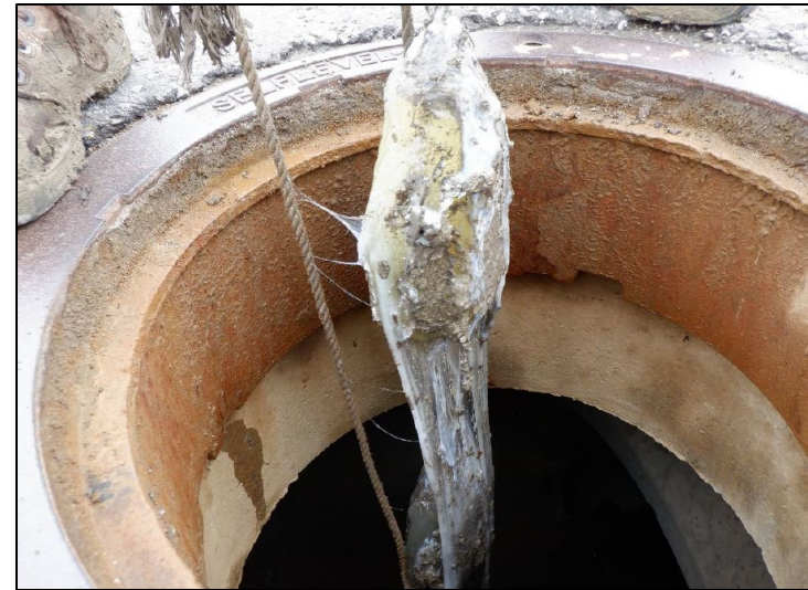
Photograph 13: Fully Spent Gel Flocculant Blocks removed from MH
