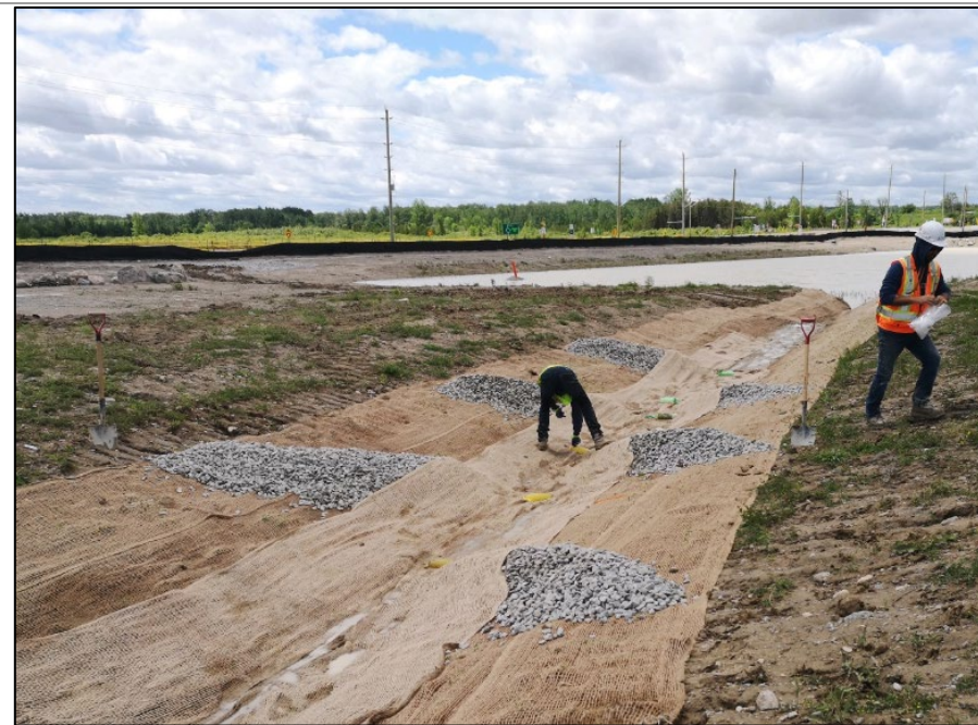
Photograph 10: SWMF #7 (east channel) with rock check dams, Treated Jute and Gel Flocculant Blocks installed
