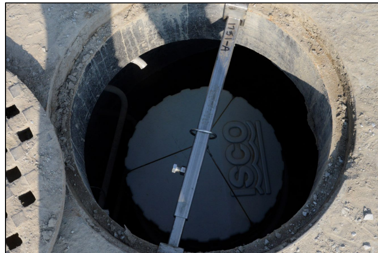
Photograph 24: Installed Autosampler Device at Target SWMF Inlet Point
