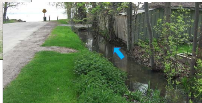
▼ Overview looking downstream near confluence with Cooks Bay; standing water and minor flow
